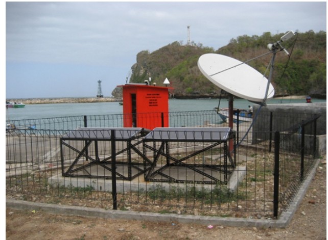
Fig. 2a. An example of a GPS-controlled tide gauge station (Sadeng, Java/Indonesia) of the GITEWS project in support of the InaTEWS system of Indonesia. The station is equipped with radar, float and pressure gauges. The GPS antenna is mounted on the top of the tide gauge hut. In addition, the meteorological sensor is visible as well as some antennas for data transmission.
