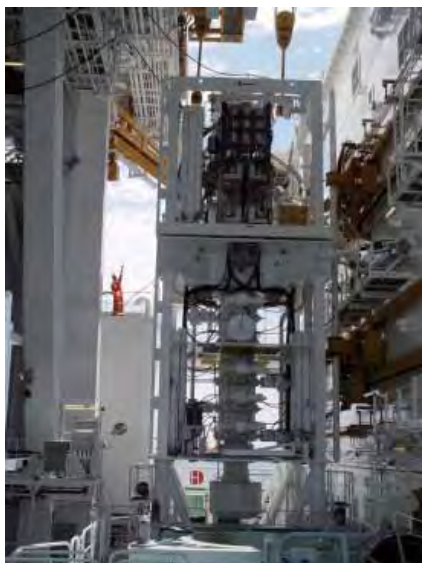
Figure 2. External view of Chikyū 's blow out preventer (BOP). BOP hangs from riser pipe attached to high-powered winches on ship's derrick and will be deployed onto seafloor through moonpool below drilling platform. Note person on left for scale.
