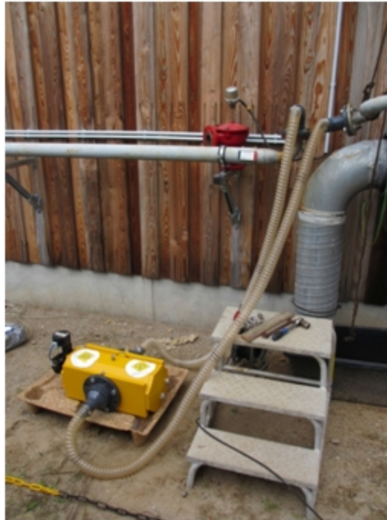
Figure 5.1.: Experimental set-up for measuring the gas volume flow rate at atmospheric conditions. The sensor was installed at the end of the flow line, temporarily replacing the flame arrester (Flammdurchschlagsventil).
