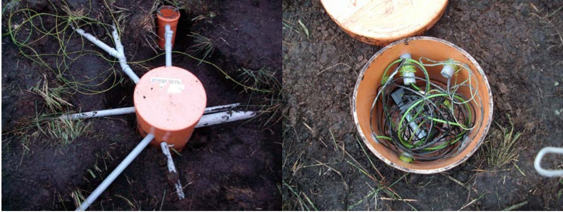
Fig. 3 Left: installation of underground cables within PVC tubes. Shown is the central location where cables from all sensors are connected to the sensor boxes. Right: Same but now with lid open and showing cables and one sensor box.
