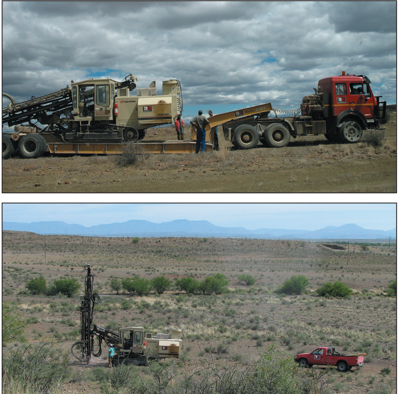
Figure 4. Field operations and instrumentation used: (a) 25 m long low-bed truck with drilling rig, (b) drilling on remote location
