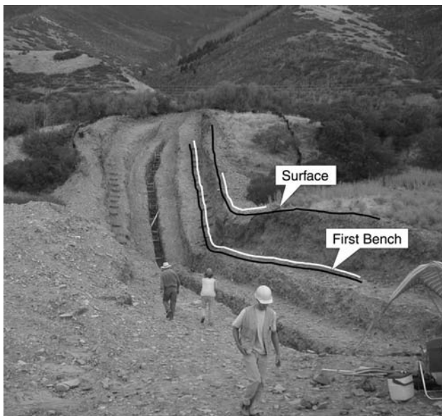
Figure 5. Photograph of the Mapleton Megatrench. The receiver lines of the seismic survey in the trench are delineated in white and the shot lines in black. The Pre-Trench seismic survey was nearly coincident with the black line along the top bench.
