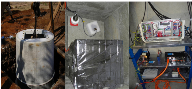
Fig. 2. Typical Vault Design - Left: GITEWS standard fibre seismic vault; Centre: station equipment with seismic sensors – broadband seismometer (in thermal insulation cover) and accelerometer; Right: electronic devices.
