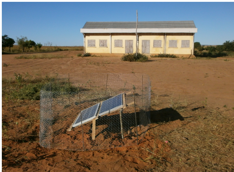
Fig. 2: Typical station installation - sensor, data logger and battery are buried for protection against daily temperature cycle and vandalism (picture shows MS04).
