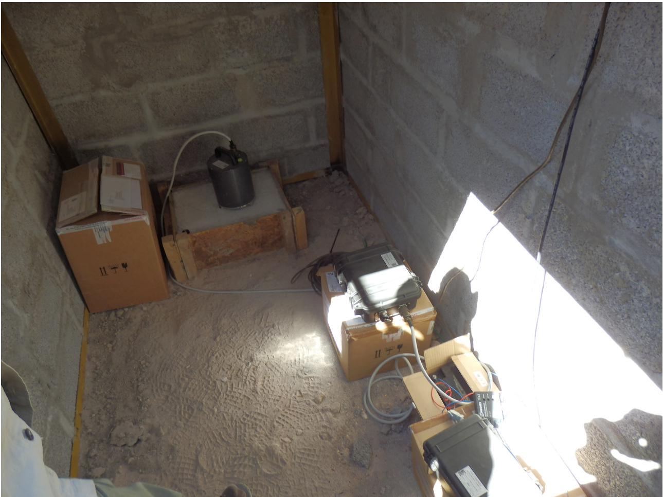
Fig. 3: Vault at station PATA, hosting a broadband seismometer, acquisition system and battery (Photo S. Cesca, November 2013).
