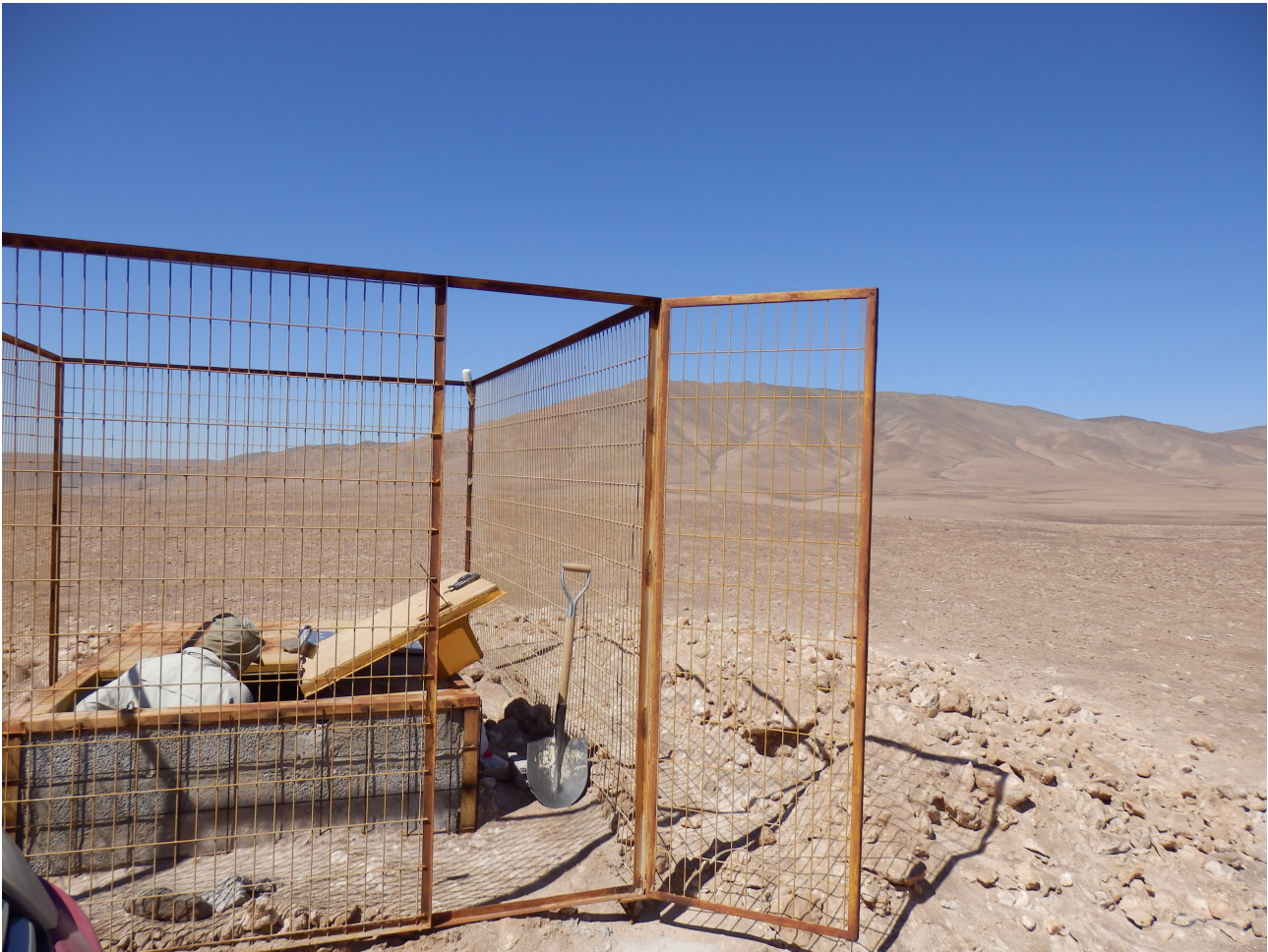
Fig. 2: View of station PATA during maintenance in November 2013 (Photo S. Cesca). The station is located in a remote site, far from any anthropogenic source of seismic noise. The installation vault is protected by a fence and a trap-door.
