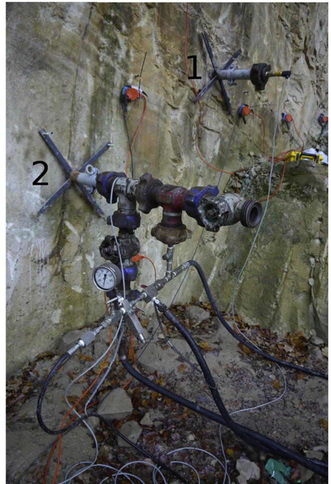
Fig. 4. Wellhead of hole 2 installed in quarry wall. Wellhead 1 was equipped with a pressure sensor. Three-component geophones were cemented into the quarry wall (red) together with piezo-elements for high frequency recording. Hole numbers are indicated.
