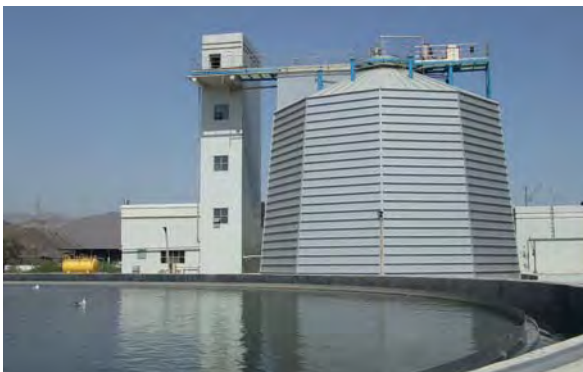
Final clarification and digester of the Fujairah treatment plant, United Arab Emirates (provided by Passavant-Roediger GmbH)
