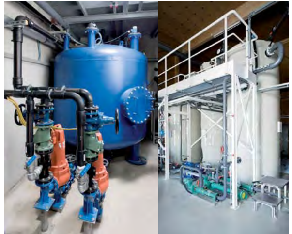
A vacuum station (left) and bioreactors in the water house
