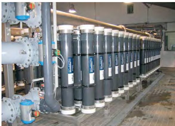
Ultrafiltration units for treating drinking water (stage 1)
