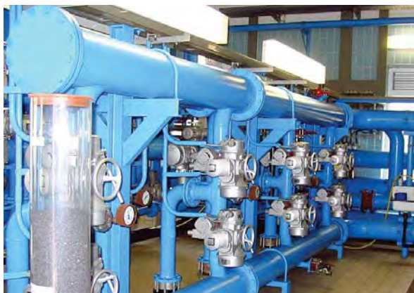
Pipes and fittings in a water works (filter outlet and flush water distribution)
