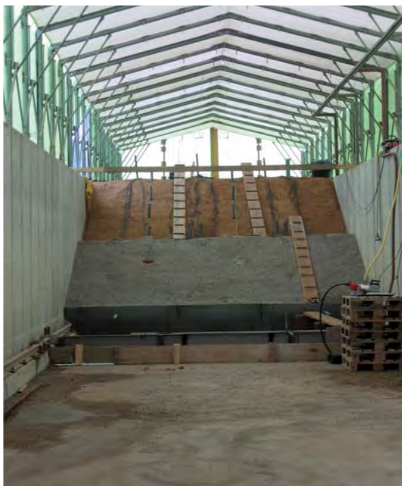
The model dyke on a natural scale (height: 3 m) proved the technical feasibility of the stabilisation procedure (viewed from land side)
