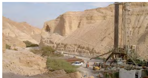
Test drilling for a well in the Judean desert near the Dead Sea as part of a research project
