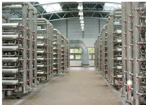
Ultrafiltration unit for treating the flush water (stage 2)
