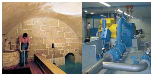
Well chamber and turbine in a water works
