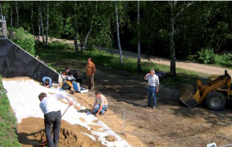
Field test on a full-scale lab dyke at the Franzius Institute of Hydraulics, Waterways and Coastal Engineering in Hanover
