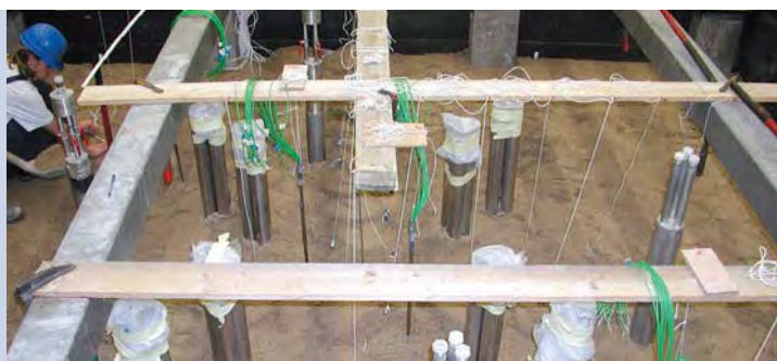
Heat lances and soil gas suction level being installed in the large tank
