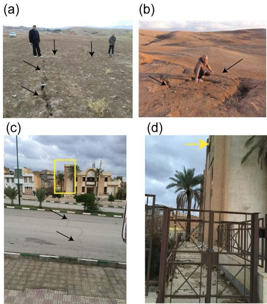
Figure 13. (a,b) Ground photos of en echelon cracks developed at P5 in Figure 9. (c) Some cracks in Qasr-e Shirin City developed along the fault (white line passing through P5 in Figure 9) that was activated in the 2017 earthquake. (d) Close-up photo of area marked by the yellow rectangle in Figure 13c. The yellow arrow marks the region of fallen bricks at the building damaged by the earthquake.
