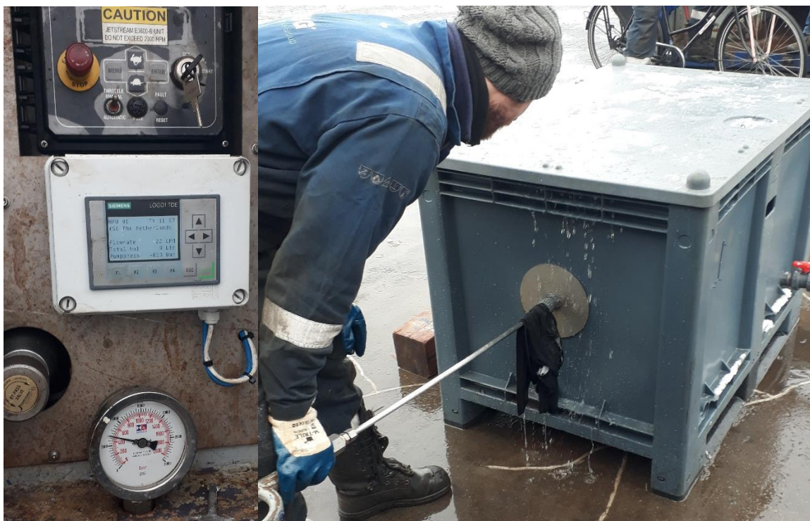
figure 46: Pump setting (left) and re-adjustment of the hp-nozzle by slightly pushing it against the rock surface
