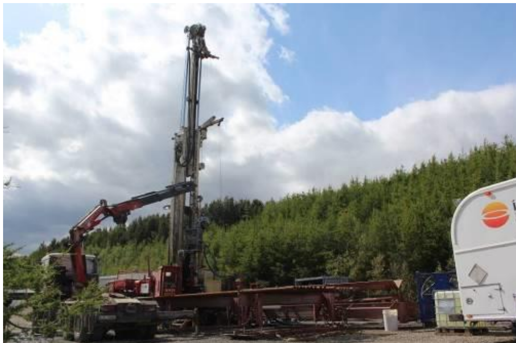
Figure 48. Drill rig Nasi, WSG coil unit and ÍSOR logging truck (picture taken in June 2019 during RJD).
