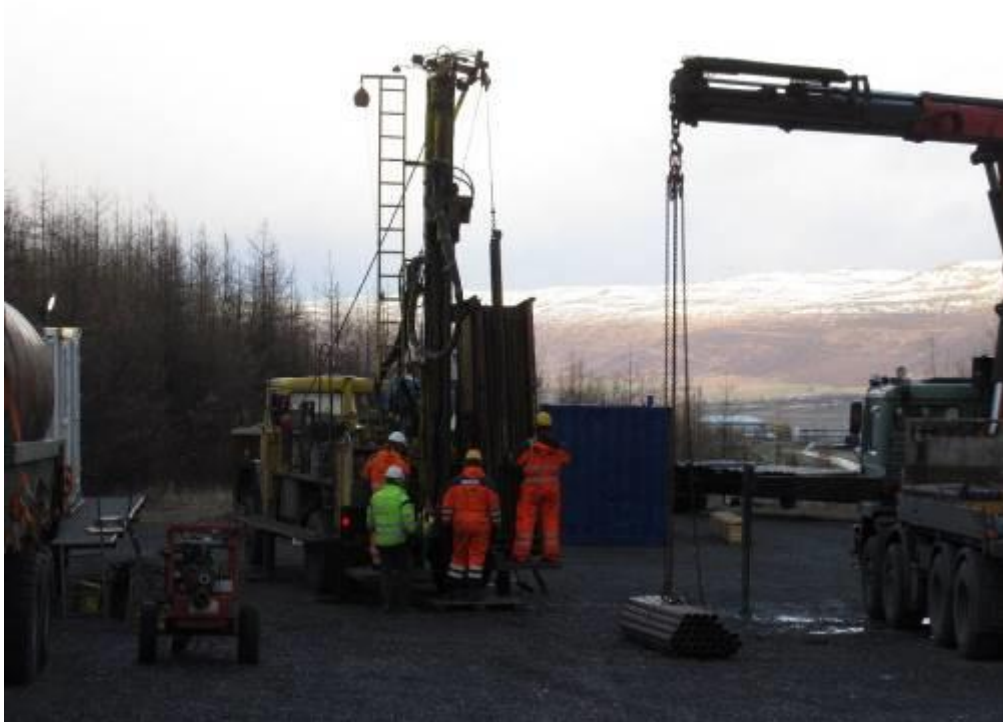
Figure 39. Drill rig "Karl Gustav" operated by RFSF. Picture taken on 19 October during RIH.
