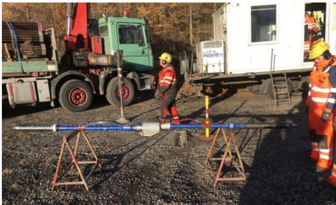
Figure 41. Bottom-hole assembly (BHA) from left consisting of geophone, decentralizing spring, deflector shoe, decentralizing spring, universal bottom hole orientation sub and crossover to NQ threads (figure by WSG).
