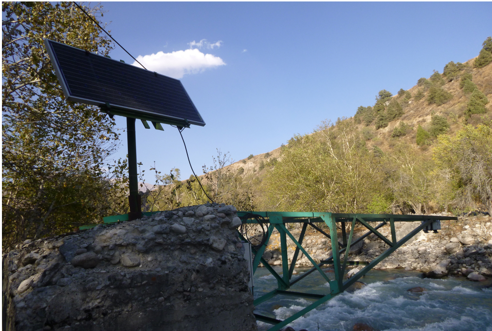
Figure 5. River discharge system at station MTAL with a solar panel and the boom for the sensor.
