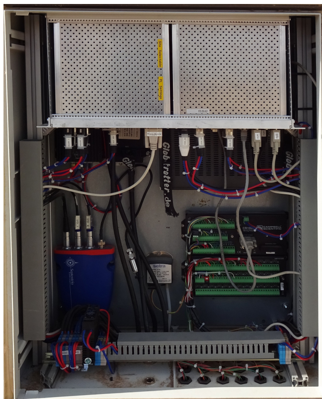
Figure 6. Station main box. Topside: the computer and power module is visible. The VSAT and Iridium modem are located at the back. Below is the GNSS receiver (left), the barometric sensor (middle) and the Campbell data logger (Schöne et al., 2013).
