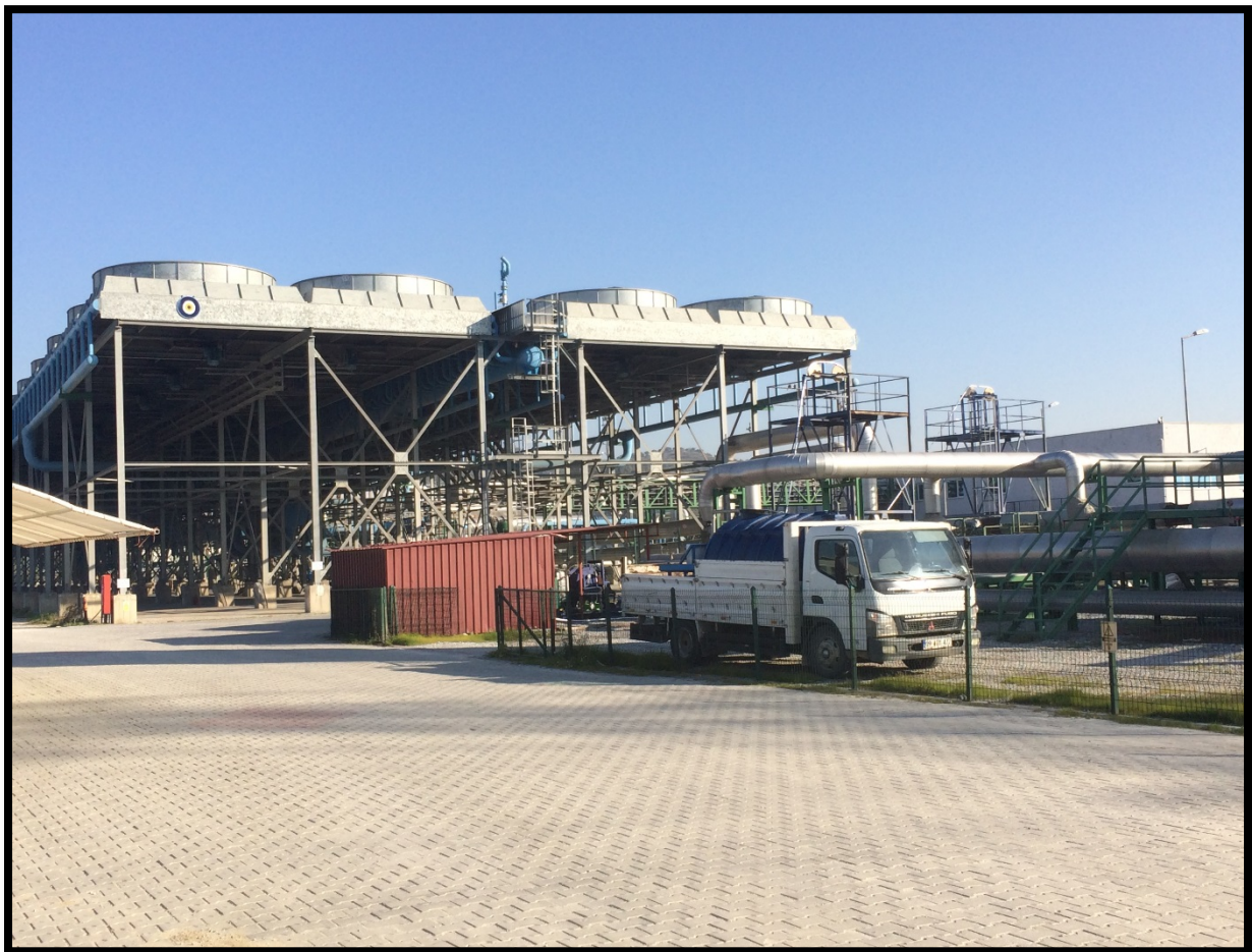
Figure 5: Surface installations of the Germencik geothermal field (GGF)
