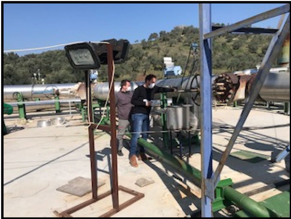
Figure 10: Sampling point in the geothermal wells
