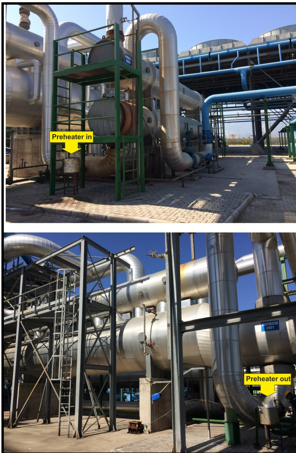
Figure 11: Sampling point in the surface equipment system (preheater)
