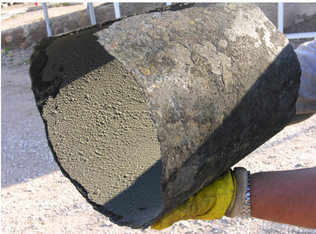
Figure 3: Silica based scaling in the Tuzla Power Plant
