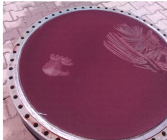
Figure 4: Stibnite scaling in the preheater system of the Germencik Power Plant
