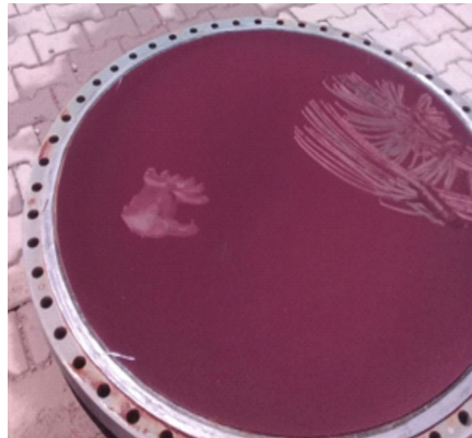
Figure 9: Stibnite scaling in the preheater system of the Germencik Power Plant
