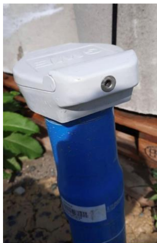
Figure 11: SEPA lockable borehole cap on top of a DN80 mm pipe.
