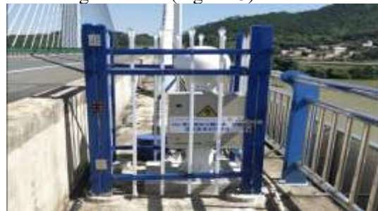
Figure 2. A GNSS monitoring point.
