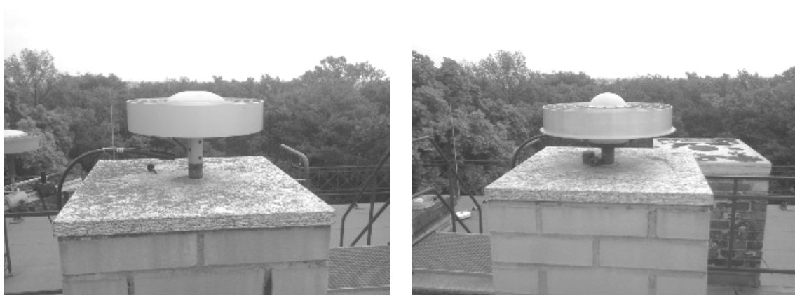
Figure 3.3: DF station POTS (left) and POTM (right) of the test network equipped with choke ring antennas.
