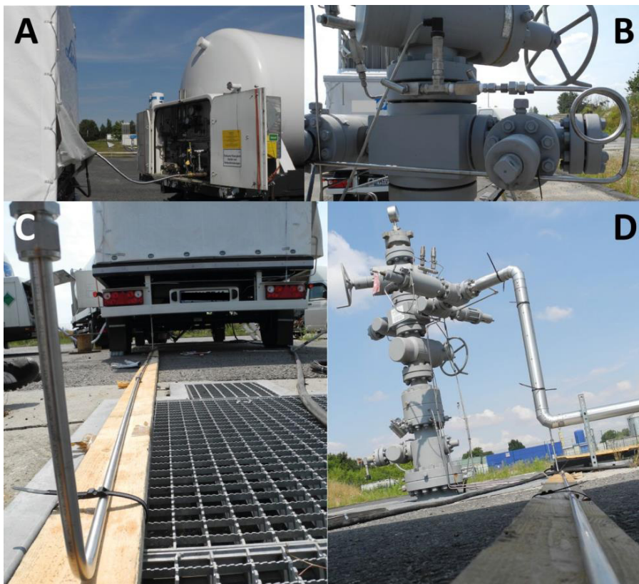
Fig. 2. A: Connection hose between N_2 storage tank and high pressure N_2 pump; B: Connection port of the stainless steel tube to \frac{1}{2} ” NPT valve at Ktzi 201 wellhead; C&D: Stainless steel tubing between high pressure N_2 pump and Ktzi 201 wellhead (Photographs by S. Fischer).
