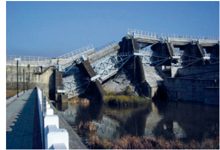
Figure 15. Affected dam after the Jiji earthquake in 1999, Taiwan
