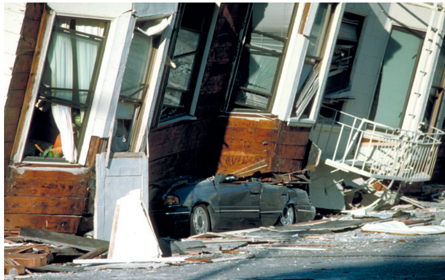
Figure 11. An automobile crushed under the third story of an apartment building in the Marina District, San Francisco—the Loma Prieta earthquake in 1989, magnitude 6.9
